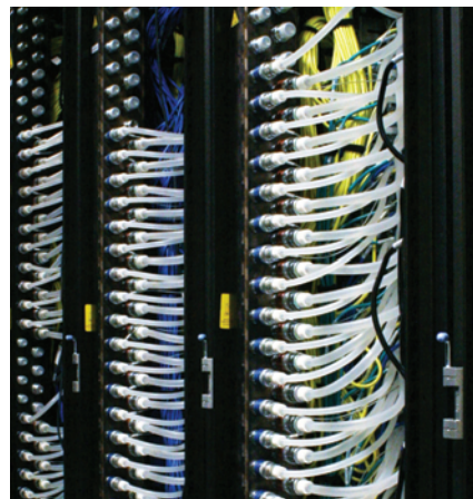
Photo 2: As part of a collaborative PNNL research project with a commercial company, fluid runs through hoses to cool a supercomputer in EMSL, a U.S. DOE national scientific user facility. This evaporative cooling technology is intended to reduce the supercomputer's heat load.
